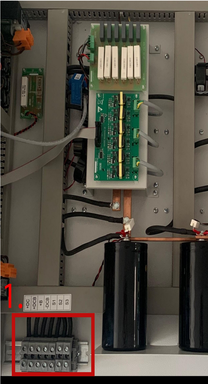
Figure 2. High power cable connection points of rectifier (port 1)
